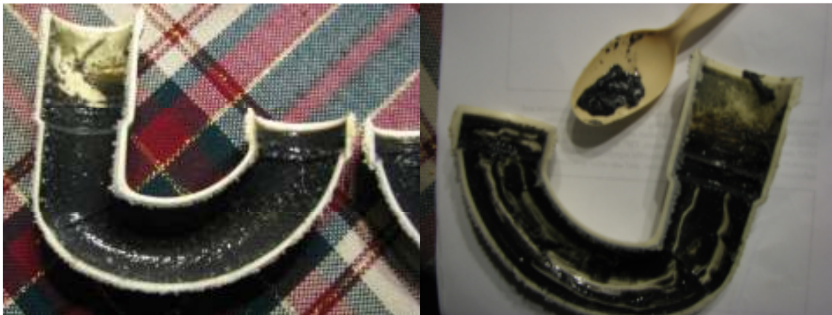
Debris Build-up in Conventional P-Trap after 1 year – breeding ground for Mold/Bacteria etc
